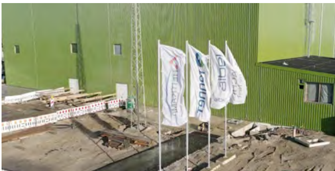
The video shows the view of the converter hall from the east, on the right in front of it the cooling plant building.
