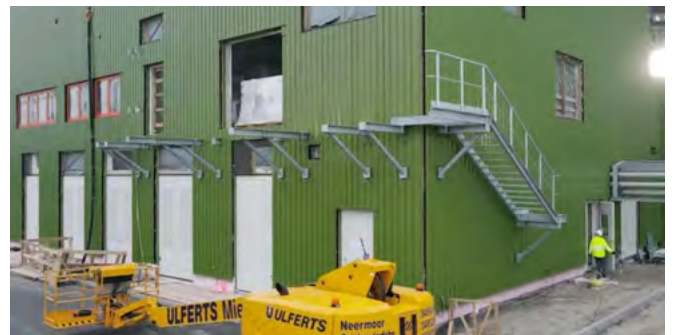
The assembly of the outer platform at the operation / service building with access to the technical rooms on the 1 st floor.
