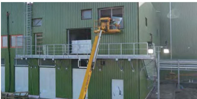
The final assembly of the facade after completion of the outer platform.
